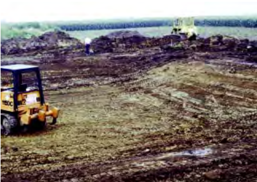
Figure 33 The sod and topsoil in a pond construction area can be stockpiled for later use
